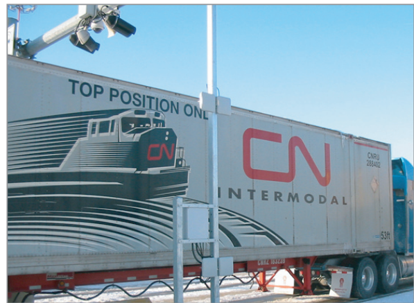
This structure designed by Bell has antenna pairs to read container level and chassis/truck cab level RFID tagged assets.
